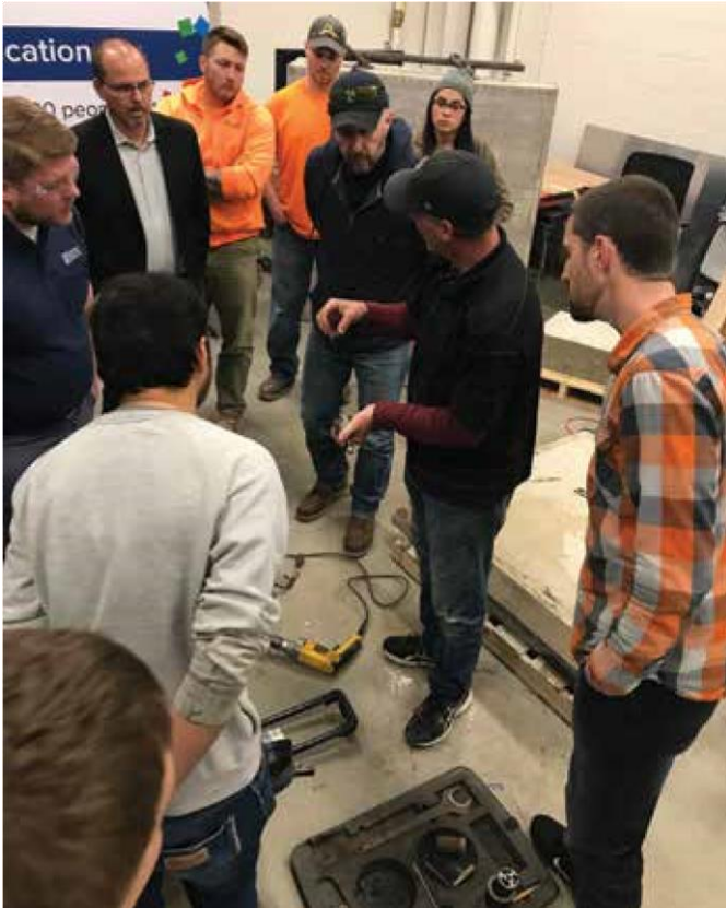
knowledge and serve as a refresher of some of the necessary knowledge Demonstration of ASTM C900, Standard Test Method for Pullout Strength of Hardened Concrete
